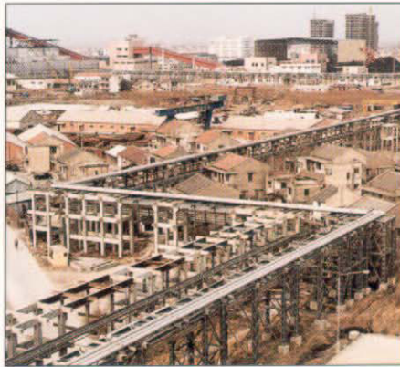
Long distance conveyor line, installed in China
